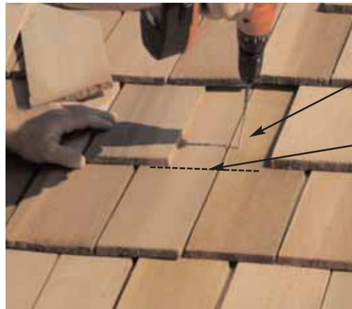
53. Screw first filler shingle down to rafters using 1 - 2 1/2" screw per panel (2 in total). Make sure to screw into both rafter.
