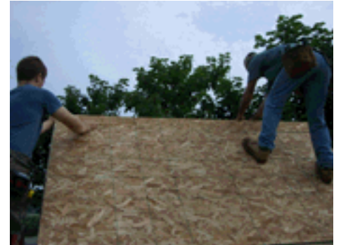
Step 16: Install ripped OSB section and fasten to rafters repeating previous steps. Repeat steps 13-16 on back roof section.
