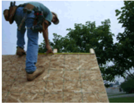
Step 15: Space rafters 2' apart and fasten OSB to rafters using 2" fasteners spaced 12" apart.
